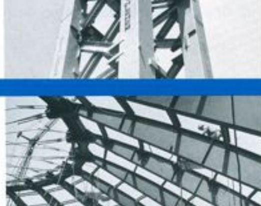
Lofty steel towers support eight giant trusses for the United States Pavilion
