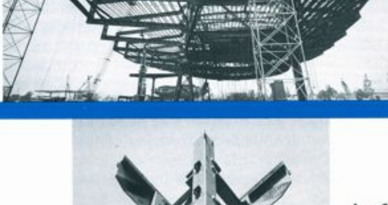
Steel U-frames connected to curving trusses frame the ride for the Bell System Exhibit
