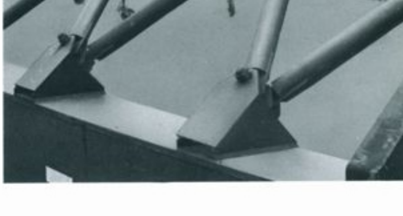
Note the braced supporting members for the carousel. Stage areas, at left, are elevated above this level and slope up toward the center well.
