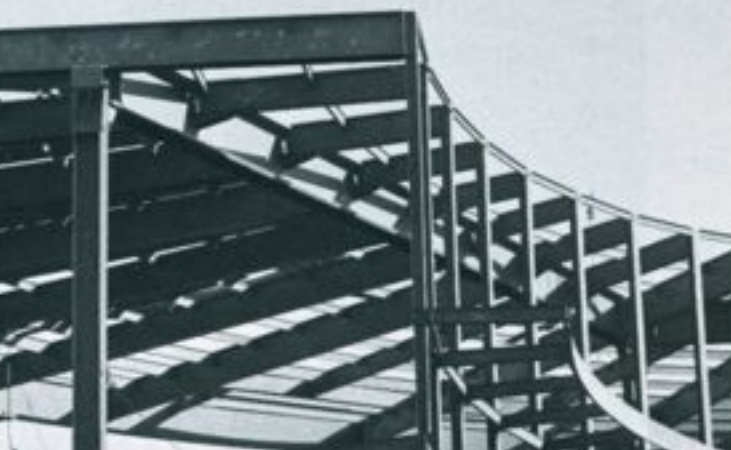
Interior steelwork, including the ring girder, was erected before the dome. The lower level of steelwork at left supports the moving theaters; the sloping beams at center support the stages; the upper level of steelwork comprises a large exhibit area.
