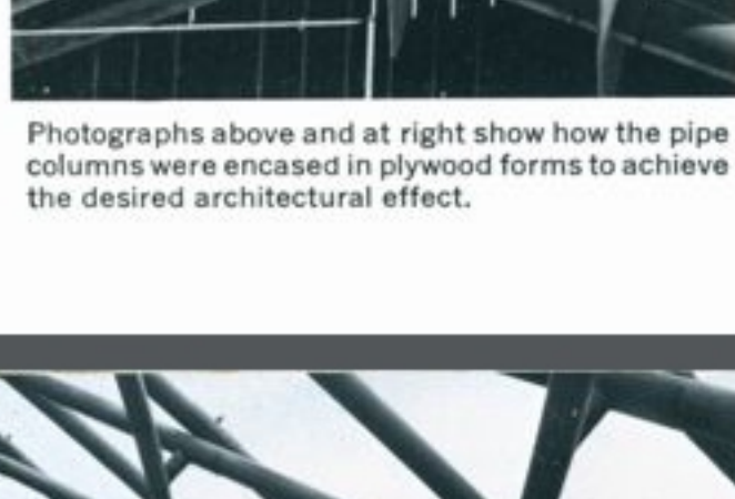
Here a decorative soffit is being applied to the all-welded ring girder, which is supported at eight points by sixteen sloping steel pipe columns, 18 in. in diameter, with 1-in. walls.
