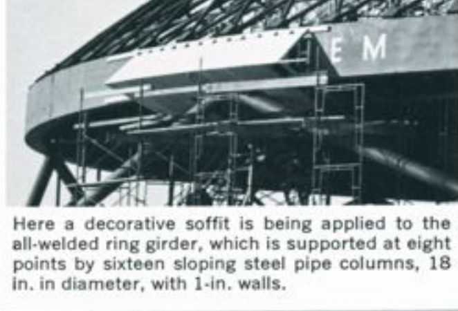
Meridians of steel tubing spring from the ring girder (bottom), and support a lower course of horizontal hoops. Formed steel decking attached to the hoops was later covered with insulation, then plywood, then a continuous silicone rubber membrane.
