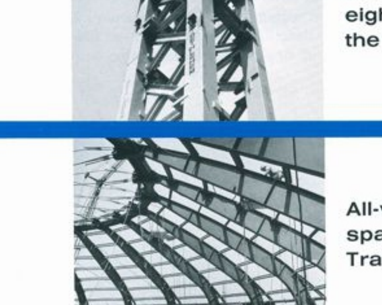
Steel U-frames connected to curving trusses frame the ride for the Bell System Exhibit
