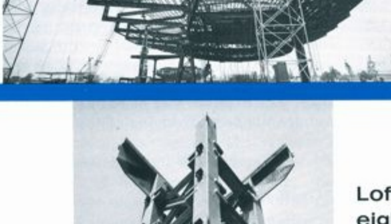
Steel U-frames connected to curving trusses frame the ride for the Bell System Exhibit
