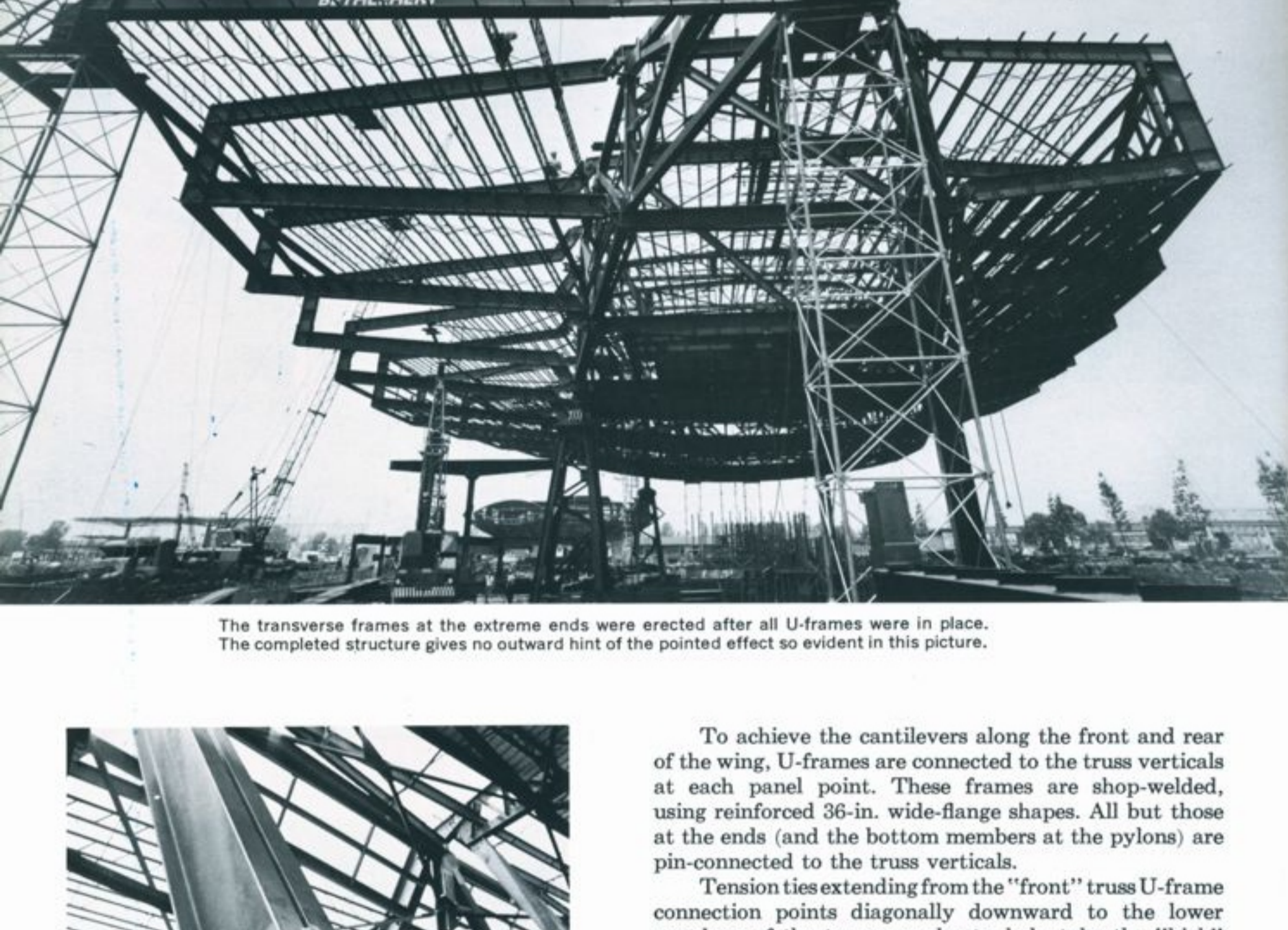
The transverse frames at the extreme ends were erected after all U-frames were in place. The completed structure gives no outward hint of the pointed effect so evident in this picture.
