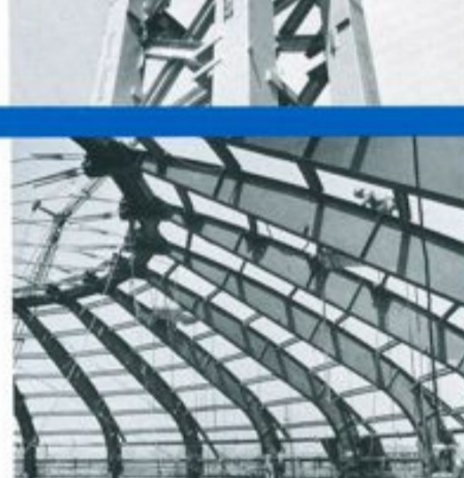
Lofty steel towers support eight giant trusses for the United States Pavilion
