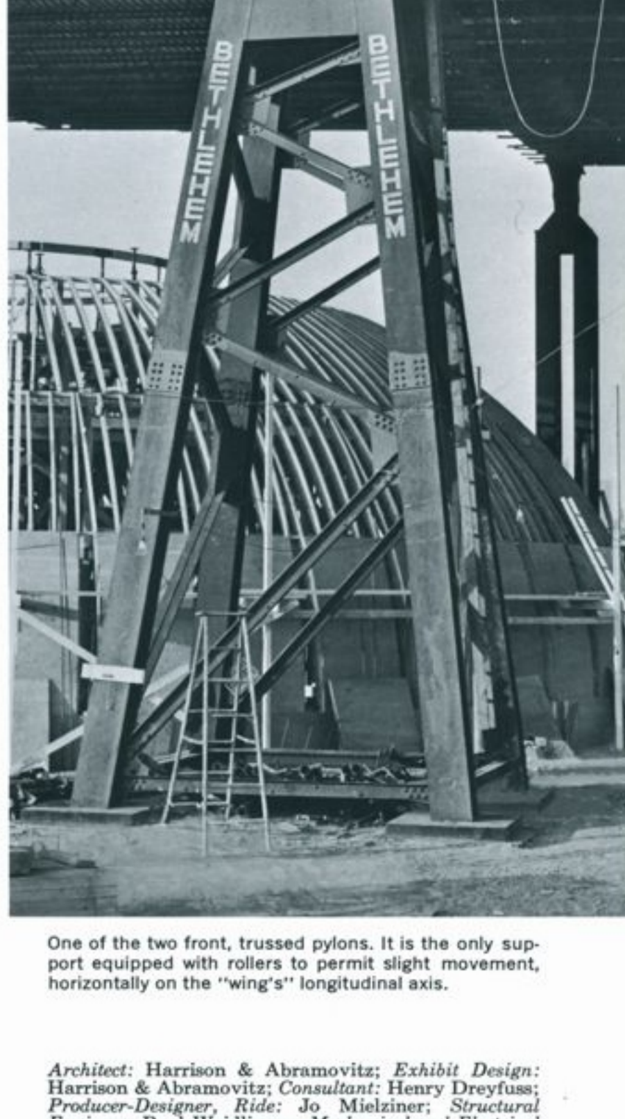
One of the two front, trussed pylons. It is the only support equipped with rollers to permit slight movement, horizontally on the "wing's" longitudinal axis.
