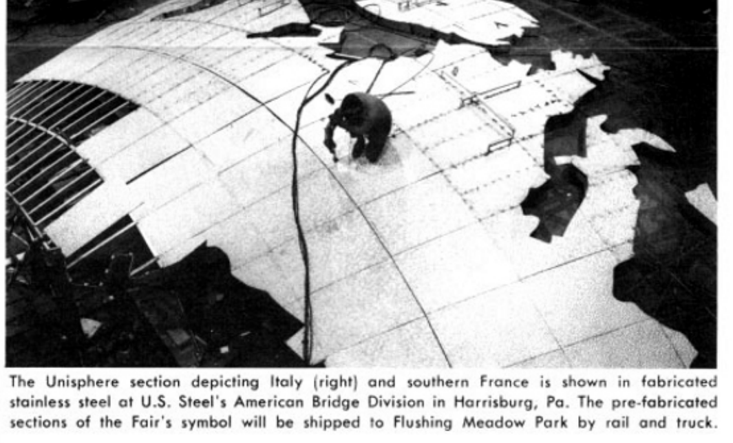
The Unisphere section depicting Italy (right) and southern France is shown in fabricated stainless steel at U.S. Steel's American Bridge Division in Harrisburg, Pa. The pre-fabricated sections of the Fair's symbol will be shipped to Flushing Meadow Park by rail and truck.
